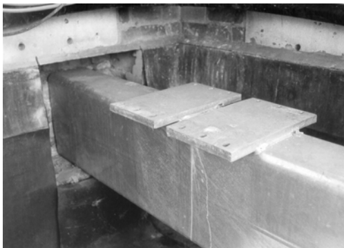
Example of steel beam designed to carry weight of carillon bellframe, set into pocket in load bearing masonry wall. Bottom of beam is approx. one foot above bellchamber floor. Note plates to receive bellframe construction.
