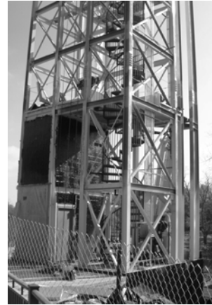
St. Hugo, Bloomfield Hills. Steel frame prior to installation of stone cladding. Note diagonal cross bracing.
