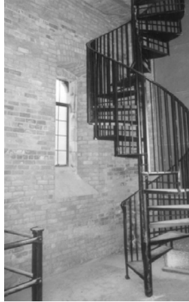
Interior view, St. Mary's of Redford, Detroit. Common brick used in masonry load bearing construction. Walls are over two feet thick. Note also spiral stair access.
