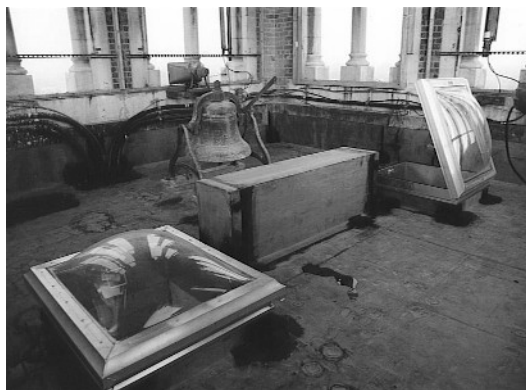
Bellchamber floor prior to installation of carillon, showing new roof hatches, curb construction for wire slot, and new rubber roof flashed around all penetrations and up side walls of bellchamber where top edge is terminated with metal counterflashing. (St. Mary's of Redford, Detroit)
